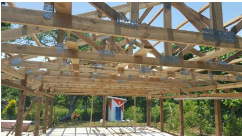
Left: Epule Kindergarten while under construction (now completed). Photo Credit: Lumu Architects & Engineers
